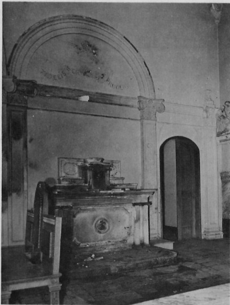
This is how the right side altar at St. Thomas looked after a fire on January 2, 1958. The fire caused more than $25,000 in damage. While the damage was being repaired, other restoration work was done on the church interior.
